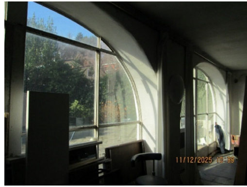
Camera condonata al piano seminterrato
