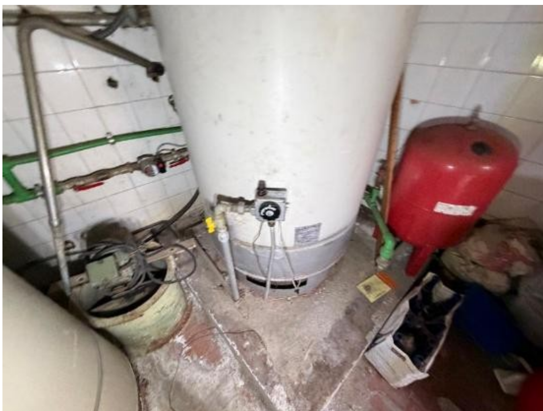
Accumulo ACS in disuso
