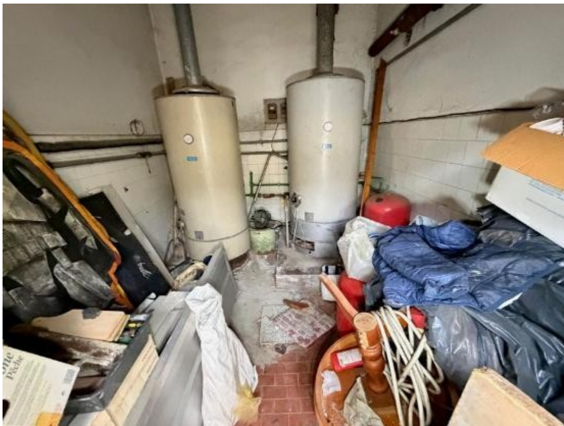
Accumulo ACS in disuso
