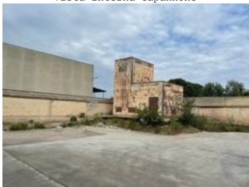
Vista cabina MT in disuso
