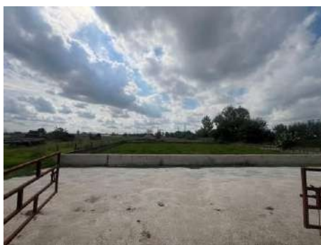
Vista 16 – Vasca liquami
