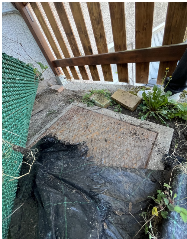
Botola cisterna gasolio
