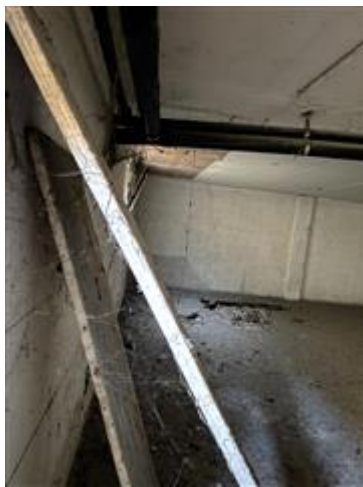
Rampa scale demolita
