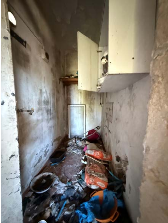
Lavanderia abusiva al piano terra (villa p.lla 256, sub. 1)
