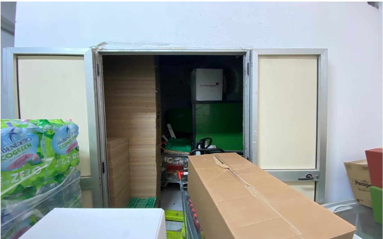
FO 30: locale macchine.
