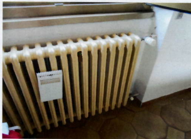
termosifoni in ghisa
