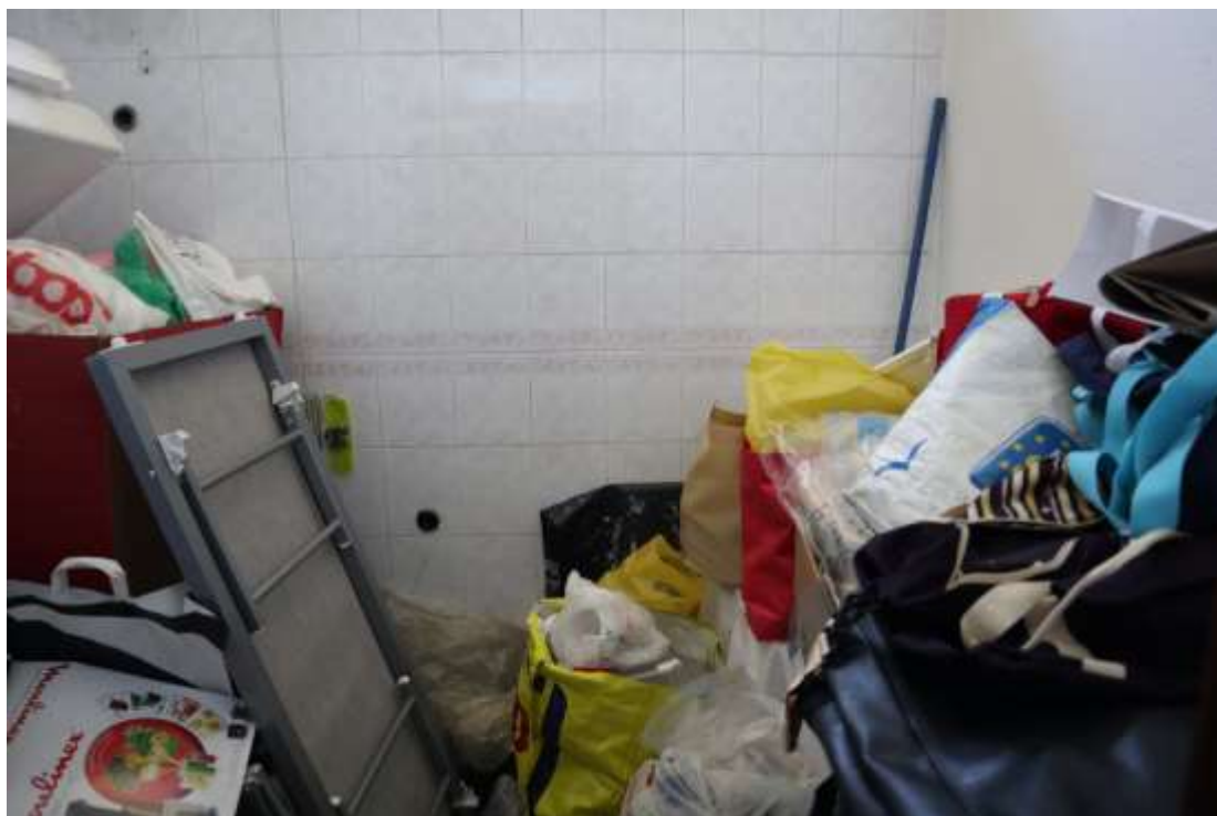
WC IN DISUSO
