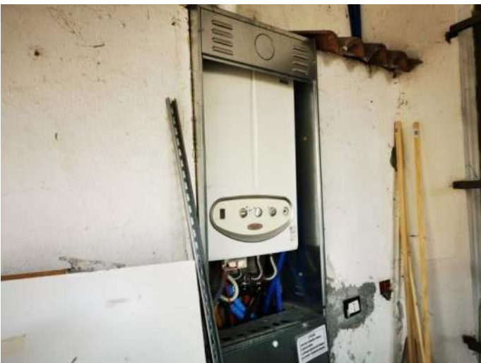
Caldaia a gas
