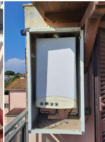
Caldaia a gas
