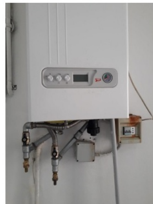
Caldaia gas part. 588 sub. 4 – via Molini 1
