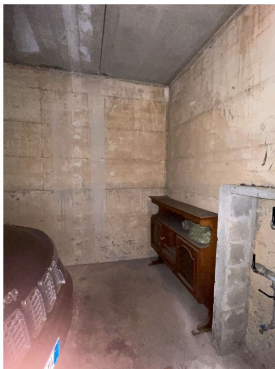
Sub.42 – locale caldaia
