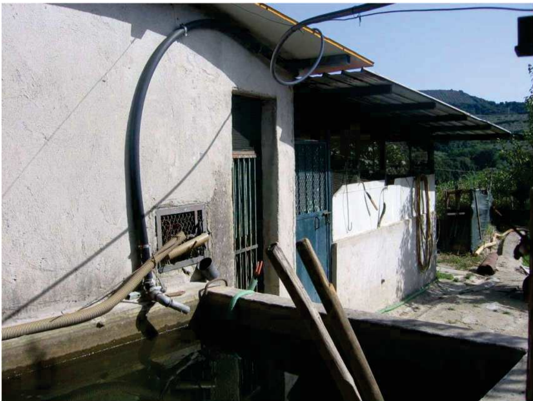
Strutture precarie abusive
