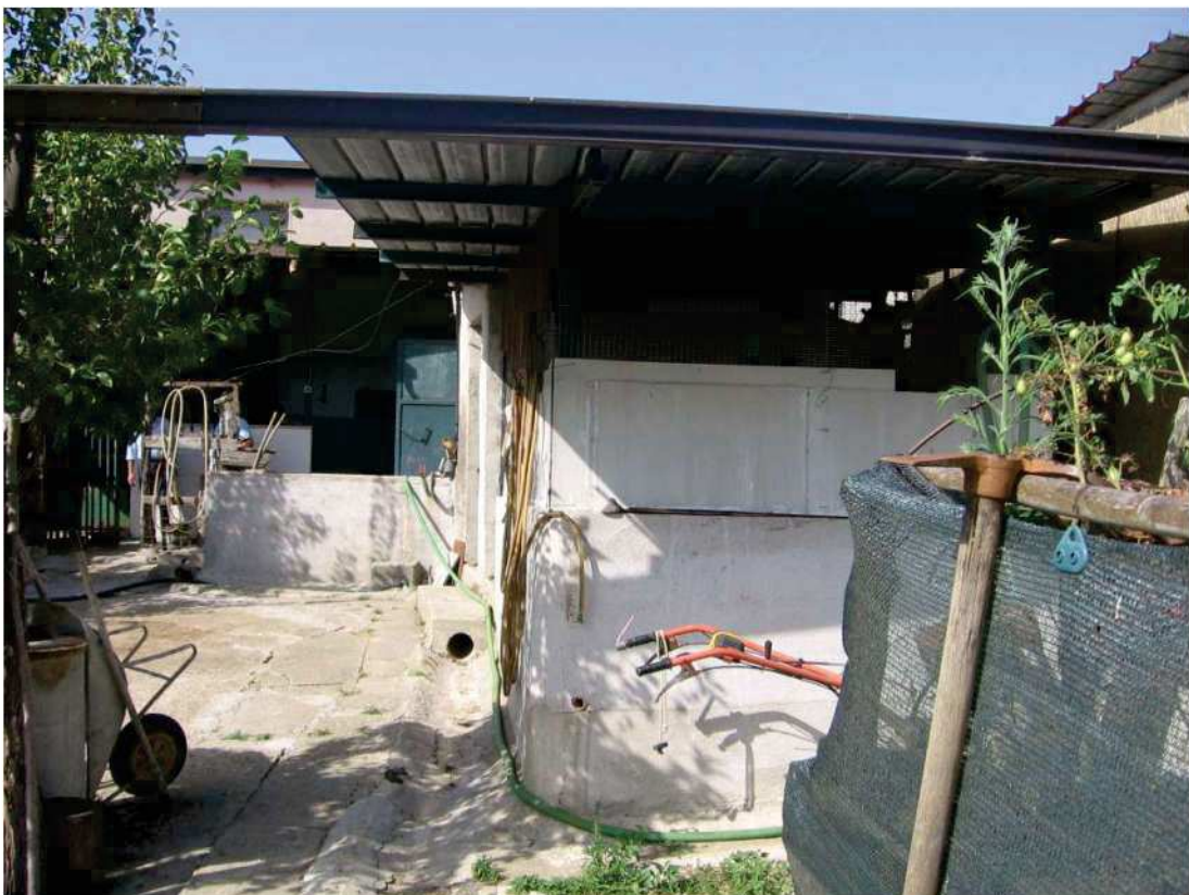
Strutture precarie abusive
