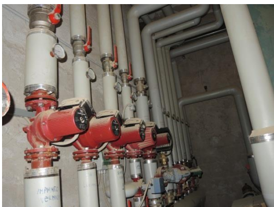
Sala pompe piano terra
