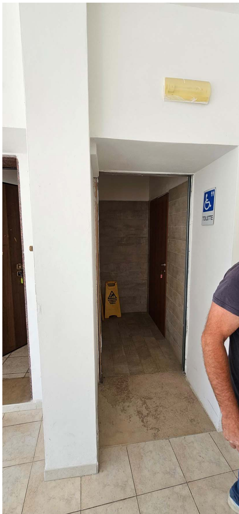
Vano difforme: bagni piano terra
