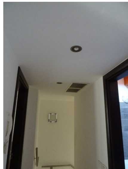
Piano 2°: Split a soffitto
