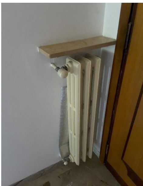
Termosifoni in ghisa
