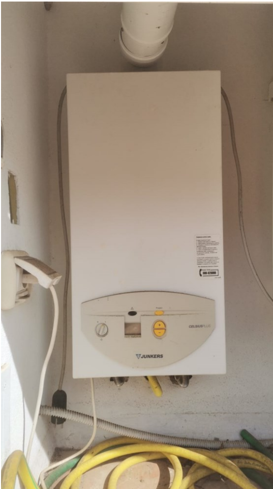
FIGURE 28: A9 CALDAIA GAS;
