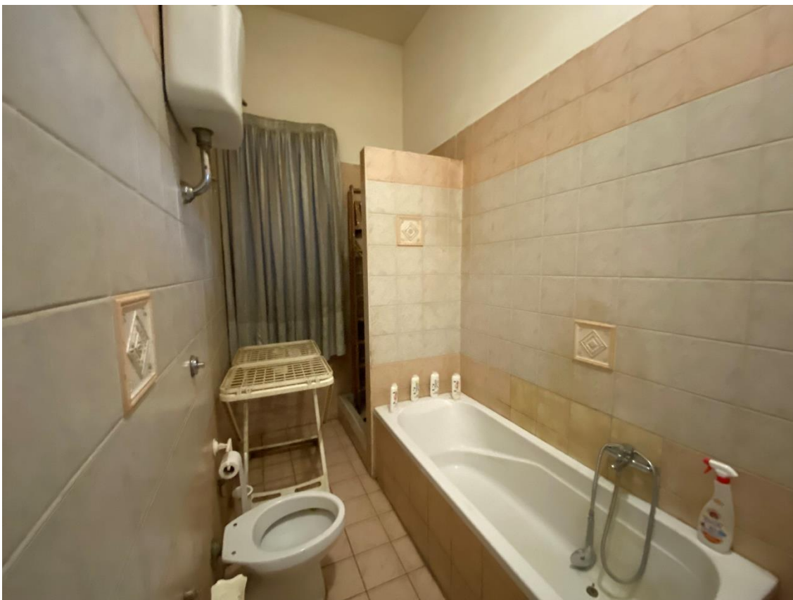
wc sub. 2 lotto 1
