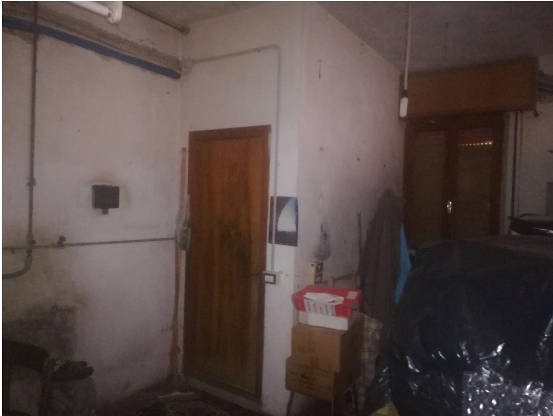
SUB. 24- PIANO TERRA : PORTA WC
